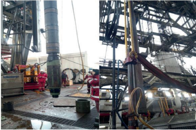
Figure 10-Transfer procedure of SSTT with rig equipment- Transfer of SSTT with using soft slings
