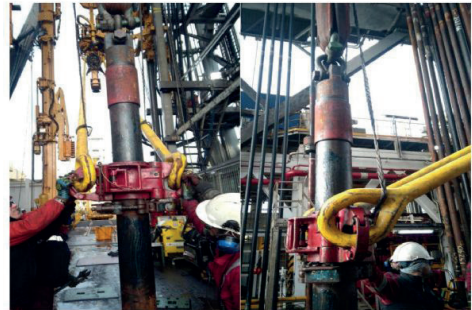
Figure 09-Transfer procedure of SSTT with rig equipment- 50' bails have been installed on MWC TDS
