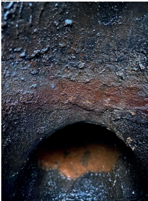
Figure 02-Scale in WT Kit after Well-5- ADJ Box - STX1 - Inlet line condition
